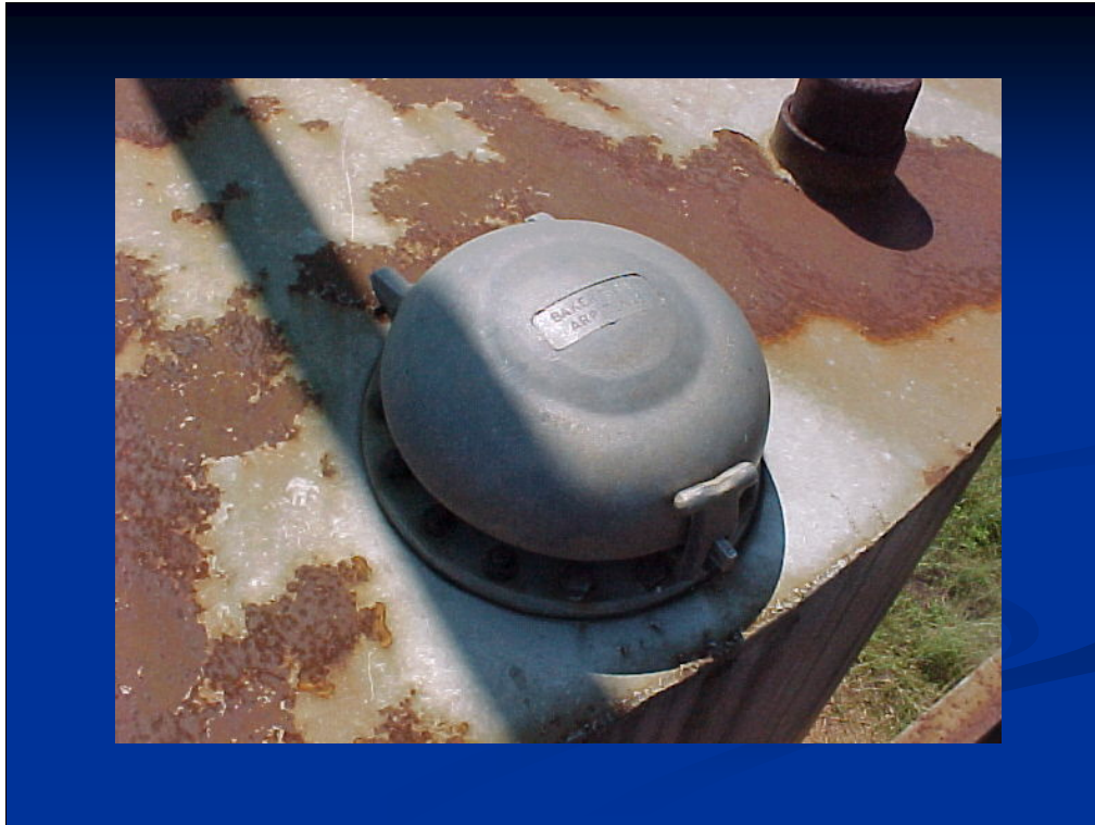
Another example of a hatch with worn out seals.
