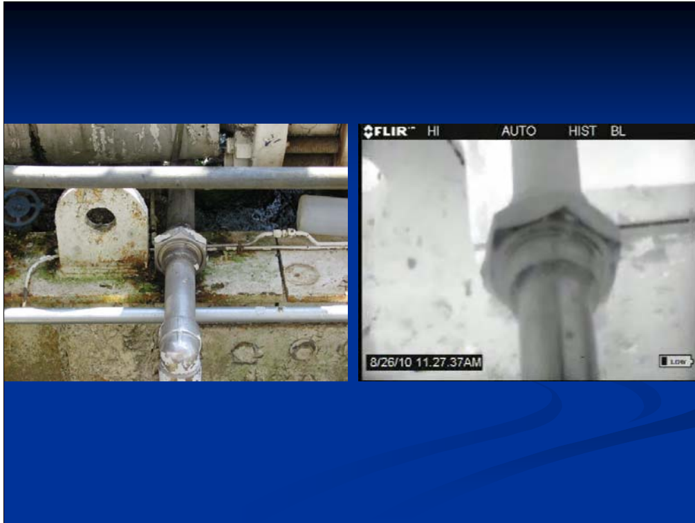
Closeup of Union Joint, previously leaking, after repair. See IR Video to the right. Leak was fixed during inspection and confirmed. No Admin Order was issued.
